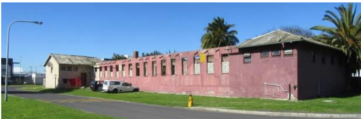
Photograph 4.9: North-facing portion of Block B which was destroyed by fire sometime late 2000 or early 2001. Block B mainly accommodates residential uses.
