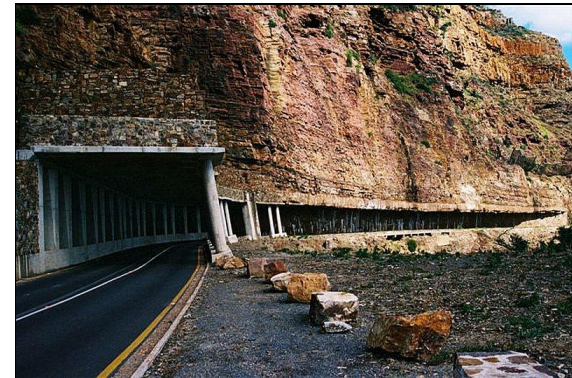
Rehab: Part of the Rehabilitation Project Led to the Construction of the Famous Half-Tunnel Canopy Structure
