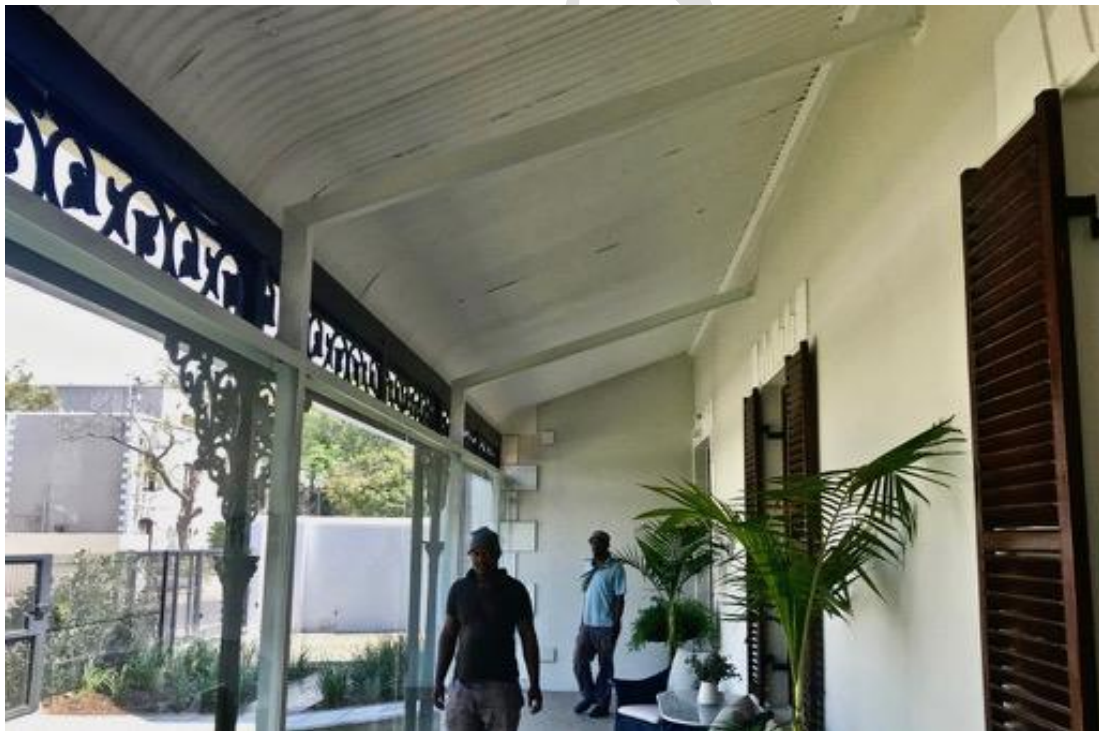
FIGURE 04: The hollow section steel members support the glazing independently of the cast iron colonnade.
