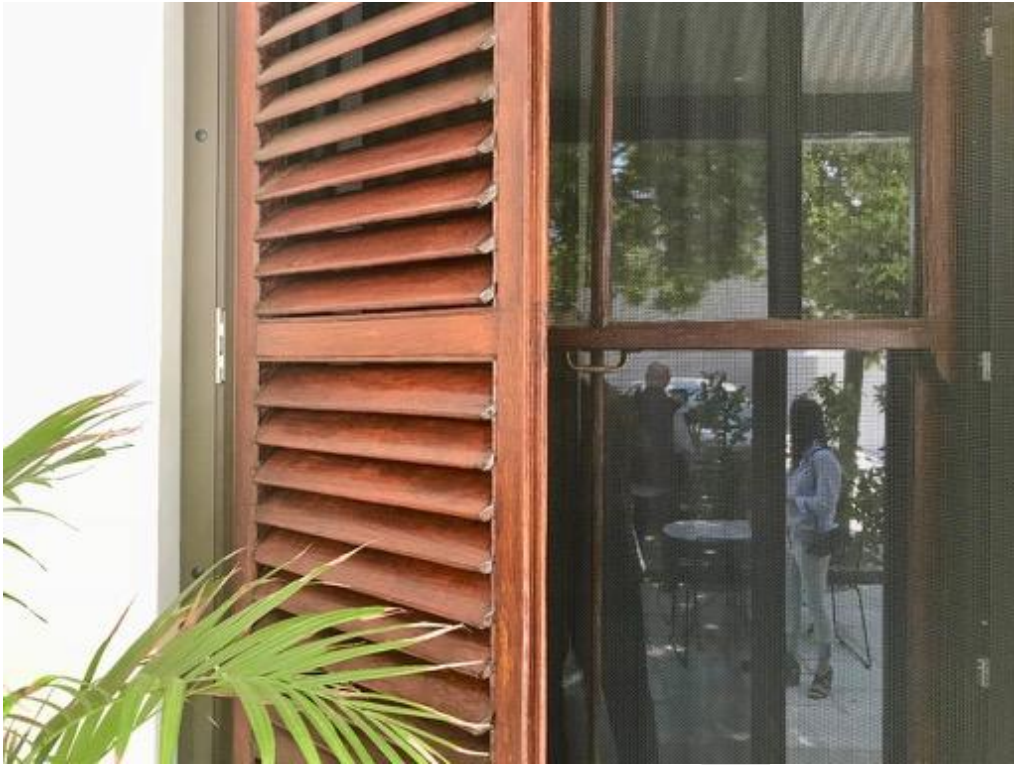
FIGURE 09: Metal mesh burglar proofing on the windows of the subject property.
