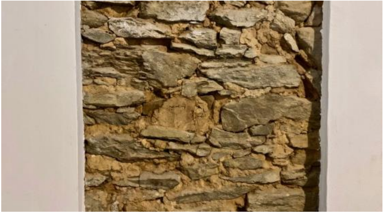
FIGURE 03: A portion of exposed wall core revealing rough stone construction bedded in a clay mortar typical of the 18 th and Earlier 19 th C.
